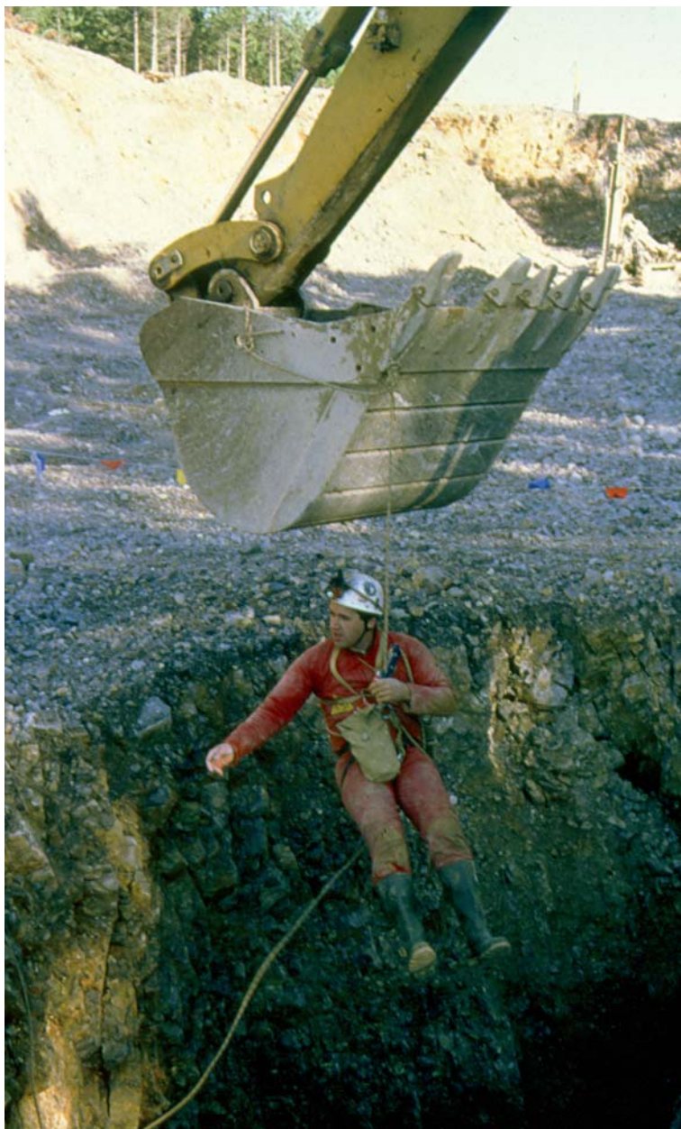
1 Raziskovanje jame, katere strop se je udrl zaradi miniranja med gradnjo avtoceste pri Divači. Research of a cave whose ceiling collapsed because of blasting during the motorway construction near Divača.
