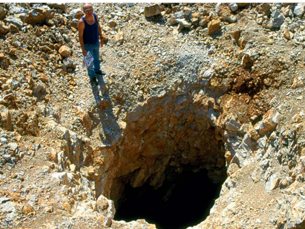
10 Udor stropa jame med gradnjo useka pri počivališču pri Divači. Collapse of a cave ceiling during the cut construction at the resting place near Divača.
