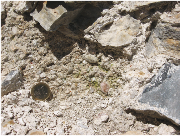
Fig. 9.12: Mortar in the inner curtain wall. The mortar was made from lime and gravelly sand from the Sava river. Brick fragments were found within the mortar. View 1.
