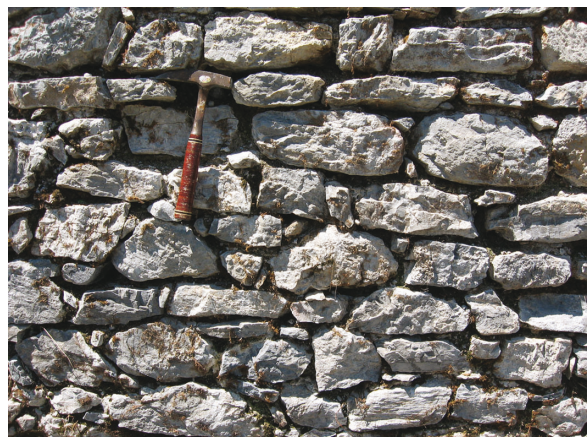
Fig. 9.16: A block of Oligocene conglomerate (OK) in the inner curtain wall. View 2.
