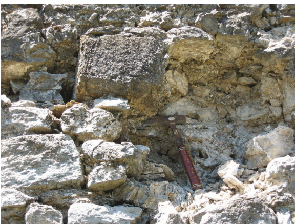
Fig. 9.15: A block of Oligocene conglomerate (OK) in the inner curtain wall. View 1.
