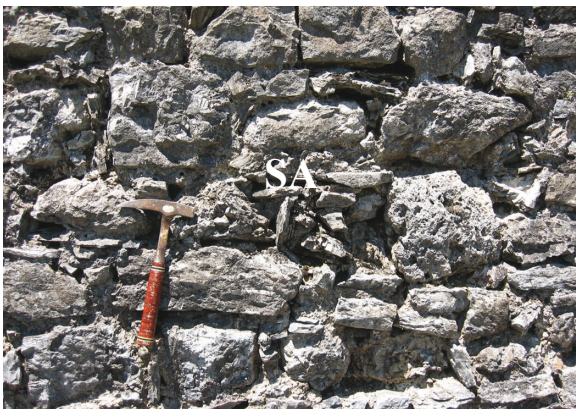
Fig. 9.10: Inner curtain wall. The stones are slightly better chiselled and provide a better fit. The blocks were chosen more carefully than in the tower and the construction was better. Fig. 9.8 shows a tufa block (L) between the quarry stones. Gaps in the wall were filled with smaller "schistose" limestone pieces (SA). View 1.
