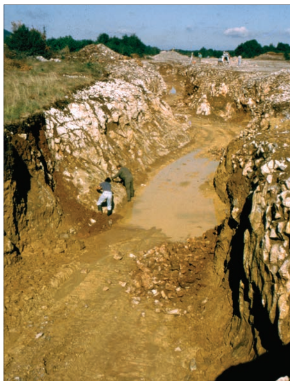
Unroofed cave discovered during road construction was filled with allogenic sediments (Photo: T. Slabe)
