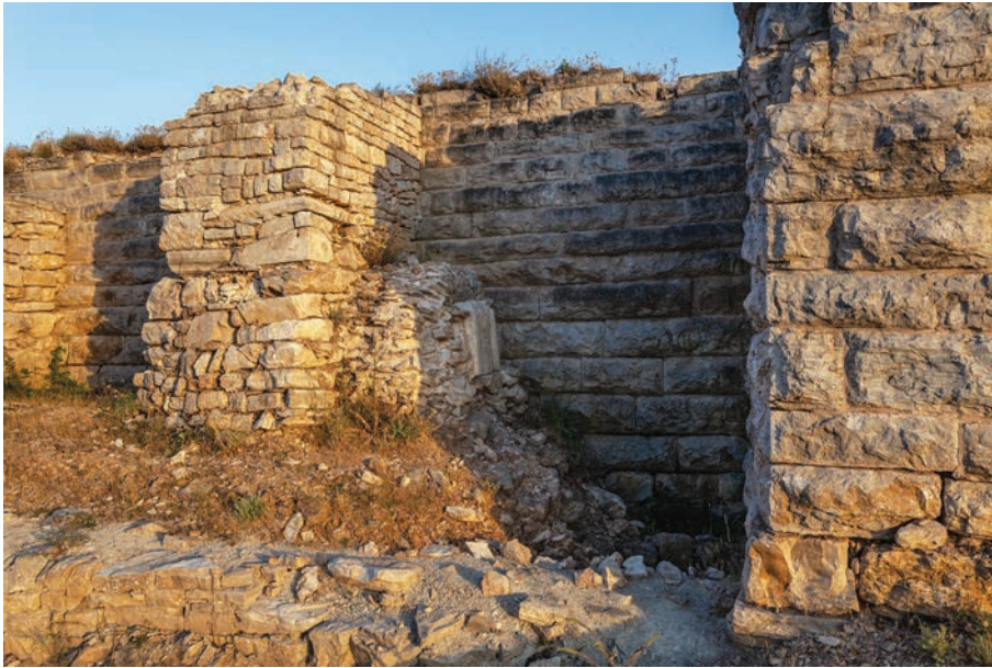
Fig. 4.10: Asseria. During Justinian's restoration, a wall buttress was built over the tomb from the first half of the 6th century (2004).
