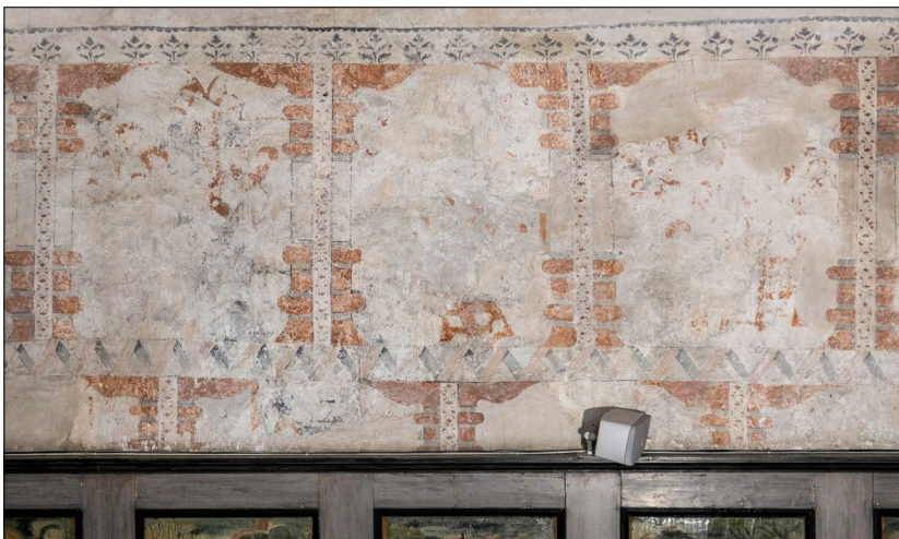
15. Stiklestad Church. Part of a frieze with fragmentary figurative scenes surrounded by reconstructed painted frames on the north wall of the nave (Photo: Susanne Kaun, 2020)
