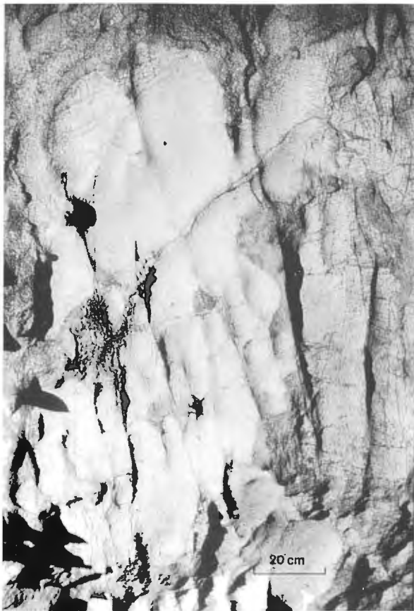
2.7.2 Scallops on the roof between Šumeča Jama and Tiha Jama, Škocjanske Jame
