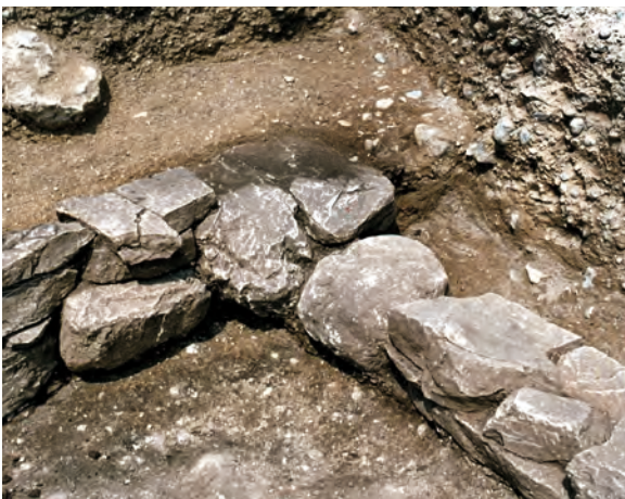
Sl. 38: Hiša 3. Gradbena faza 1. Severni vogal temeljnega zidu; pogled z juga. Fig. 38: House 3. Construction Phase 1. North corner of foundations; view from the south.
