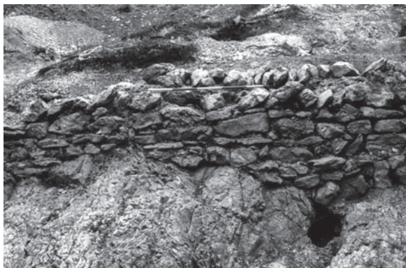
Sl. 2.17: Stavba 1, zid 3 – notranje lice. Detajl osrednjega dela zidu. Fig. 2.17: Building 1, wall 3 - interior. Detail of the central part.
